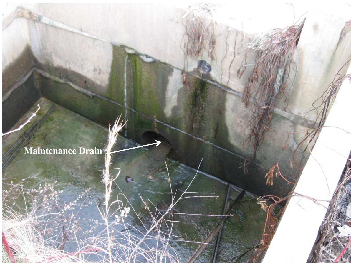
Figure 5.3 Draining Pond with Maintenance Valve
