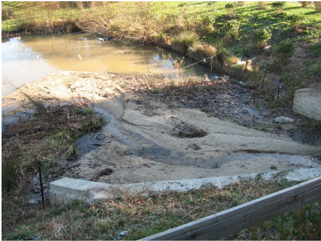
Figure 4.4 Sedimentation in Forebay
