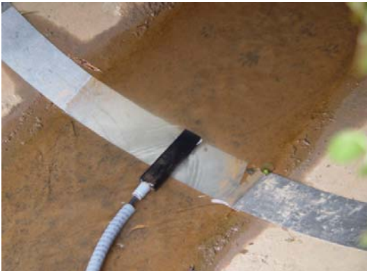
Figure 1: Area velocity meter installed in culvert
