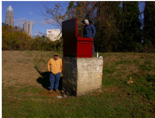
Figure 1: Outlet Structure at Morehead Dry Detention Basin.
