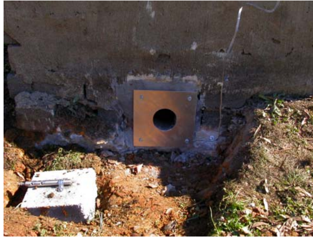
Figure 2: Orifice Plate installed at Morehead Dry Detention Basin.
