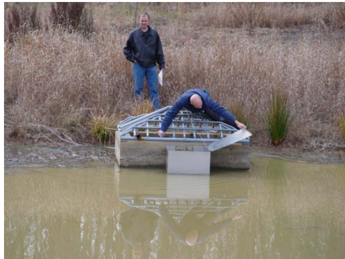
Figure 1: Edward's Branch Outlet Structure with Debris Screen
