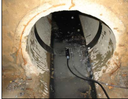
Figure 2: Typical installation of area-velocity probe (left) and sampler intake (right) with expansion bracket
