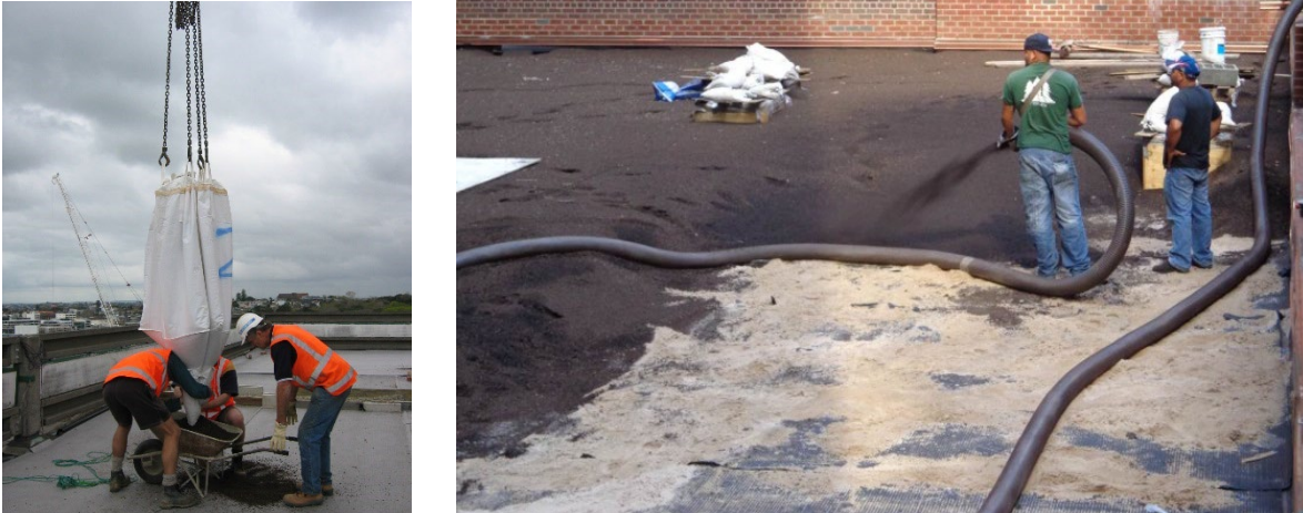
Figure 11. Growing media installation by crane hoist (left) and pneumatic blower (right) (Dr. Elizabeth Fassman)
