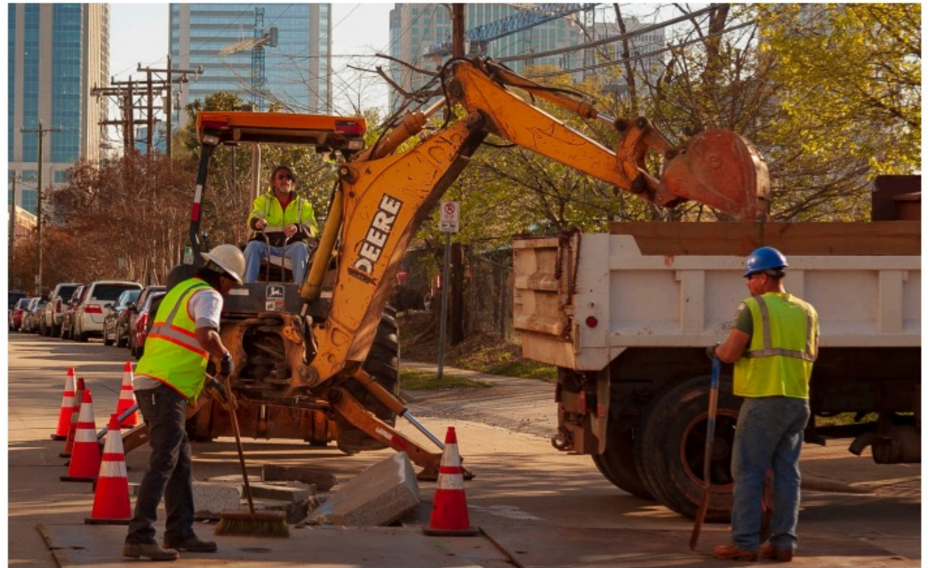
Crews dig at strategic locations reducing the amount of lane closures, pavement repair, and inconvenience to customers.
