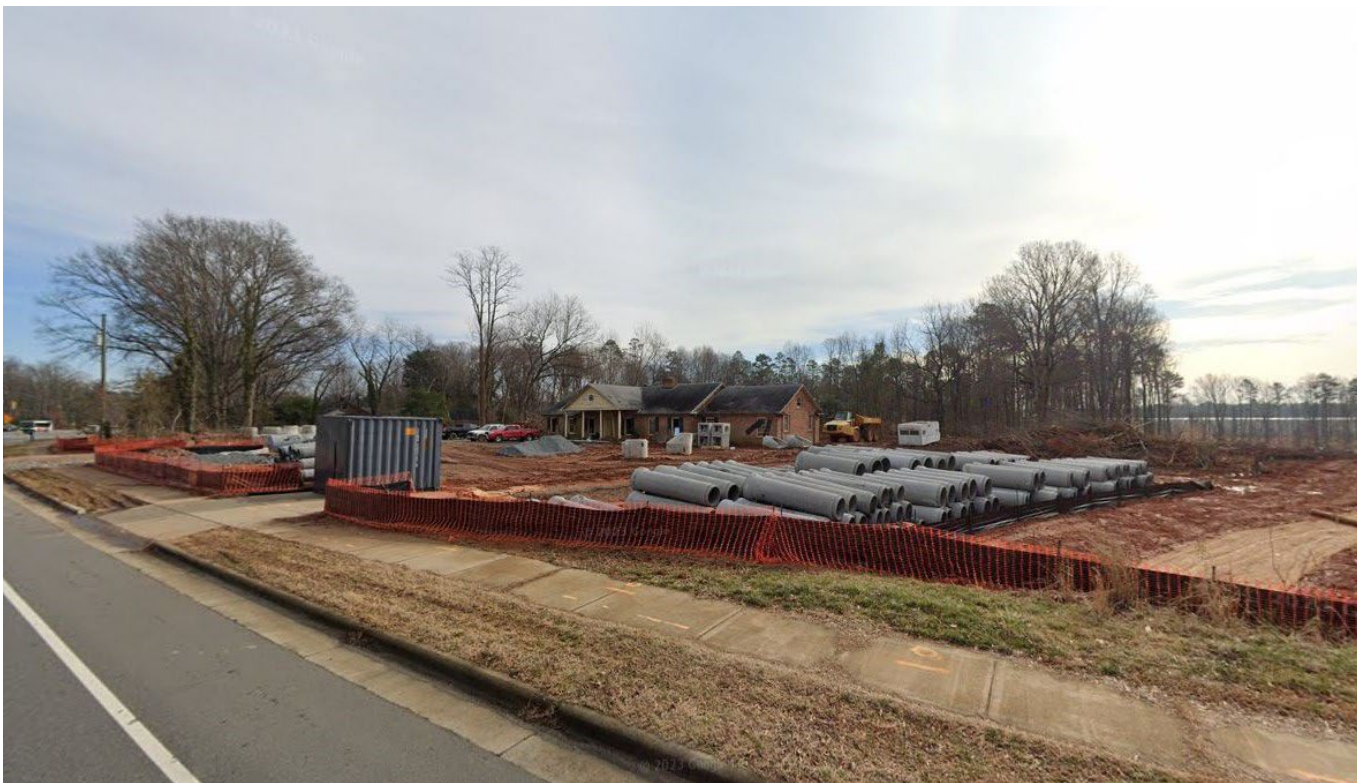
View of a townhome development under construction to the north of the site along Mallard Creek Road.
