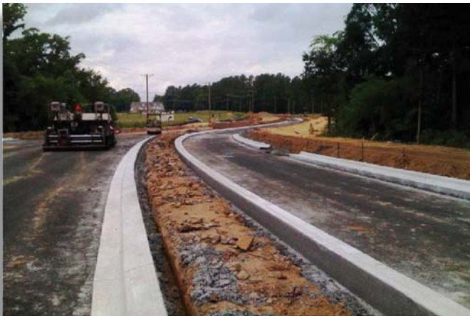
The Shopton Road West re-alignment will address congestion and improve safety in the Steele Creek area.
