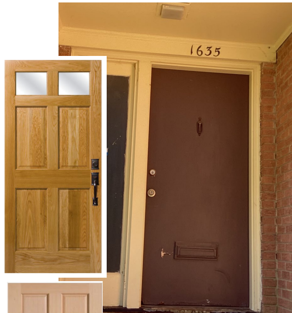
Non-Original Front Door Change. All wood panel door.
