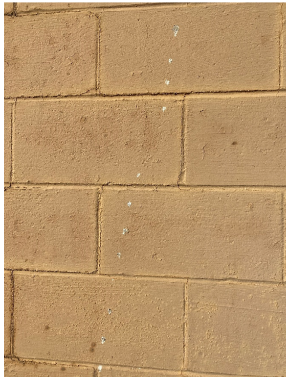
Picture #4 – Minor Cracking
