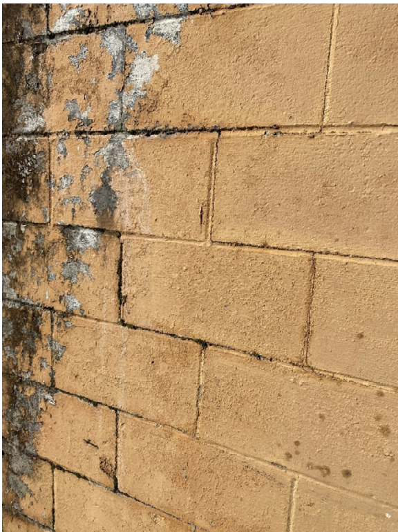
Picture #3 – Minor Cracking
