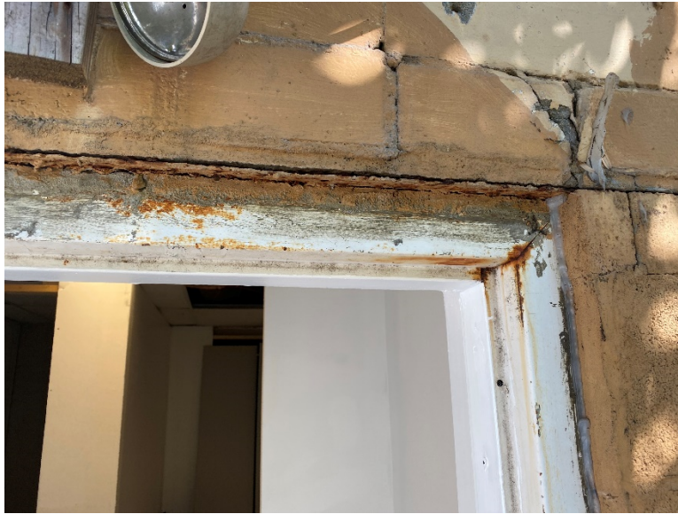
Picture #5 – Lintel Rust and Cracks
