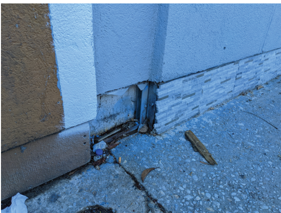
Compromised exterior envelope
