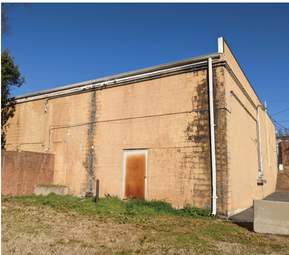
Water stained exterior
