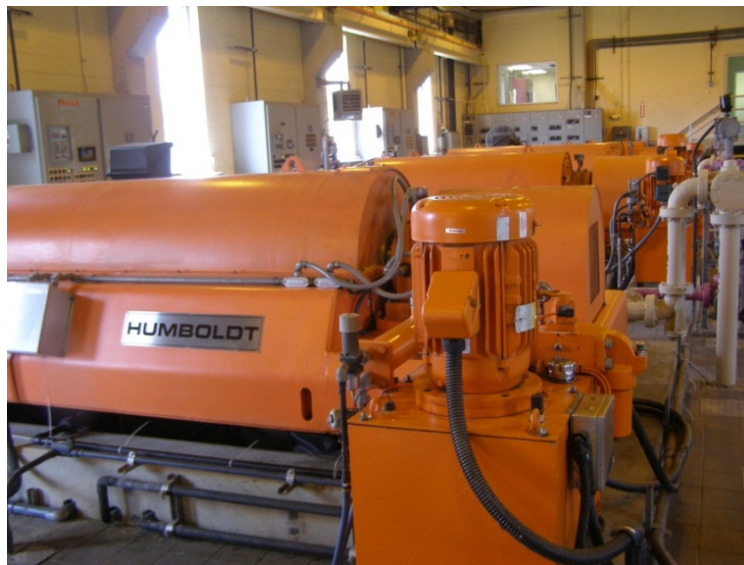
Figure 4-17 Thickening and Dewatering Centrifuges
