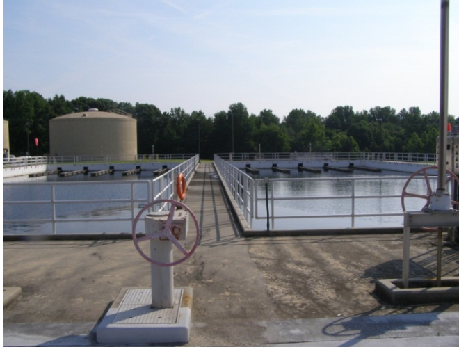
Figure 2-10 Lee S. Dukes WTP Sedimentation Basins
