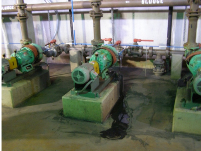
Figure 2-7 Vest WTP Unthickened Residuals Pump
