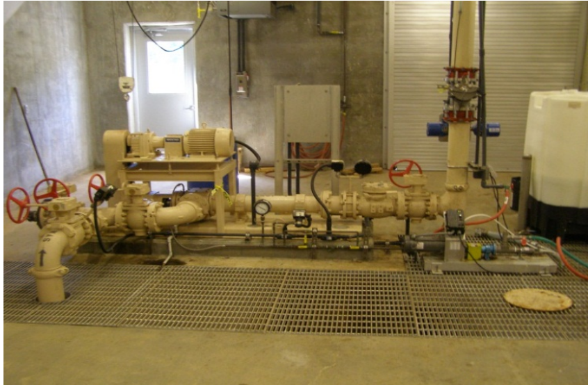
Figure 4-15 WAS Pumping System
