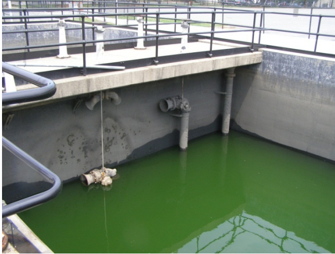
Figure 2-8 Vest Decant Tank
