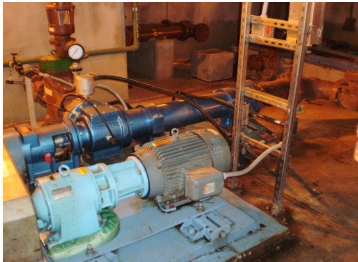
Figure 4-12 Primary Sludge Pump
