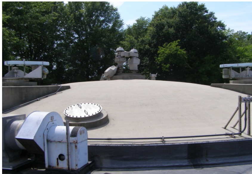
Figure 4-20 Anaerobic Digester with Fixed Cover
