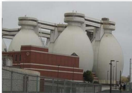
Figure 8-3 Egg-Shaped Anaerobic Digesters
