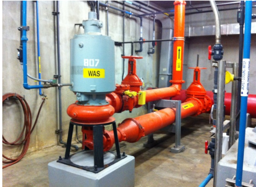
Figure 4-3 WAS Pump for Thickening Centrifuge
